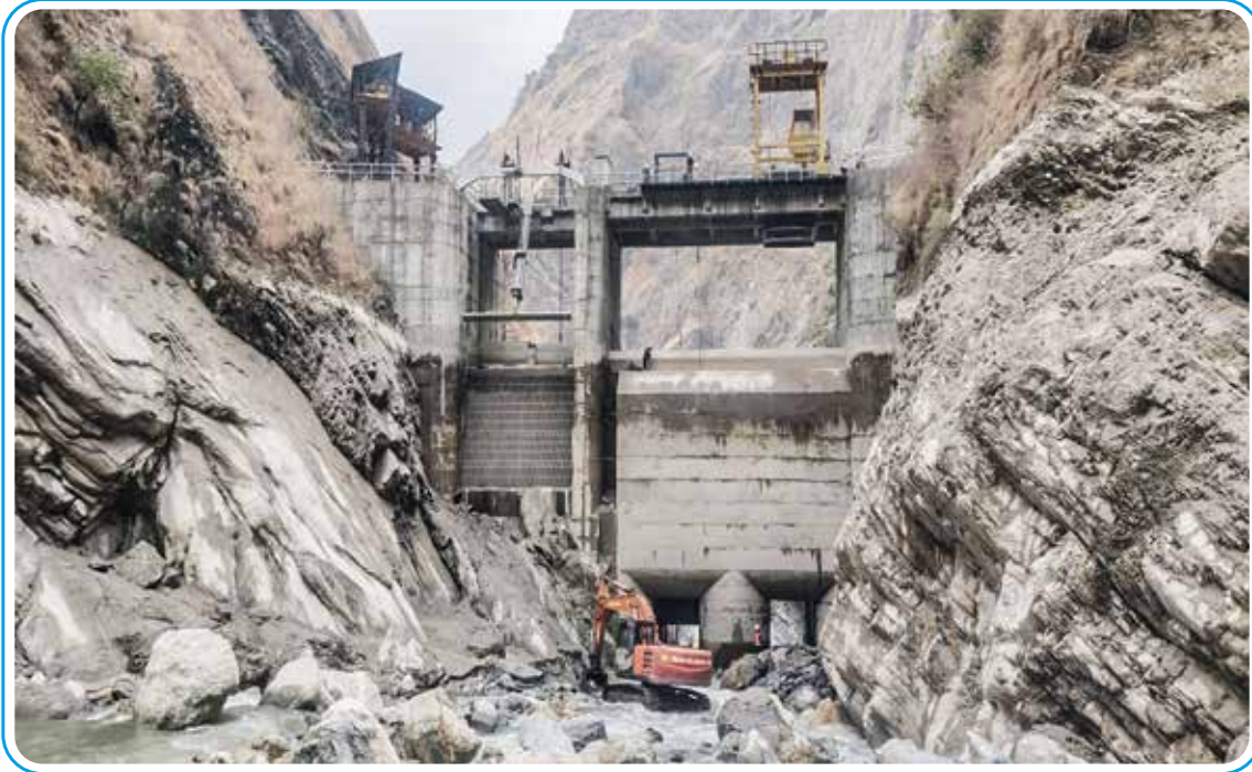
River diversion for Under sluice sill beam repairing Work of Mistri Khola HEP
