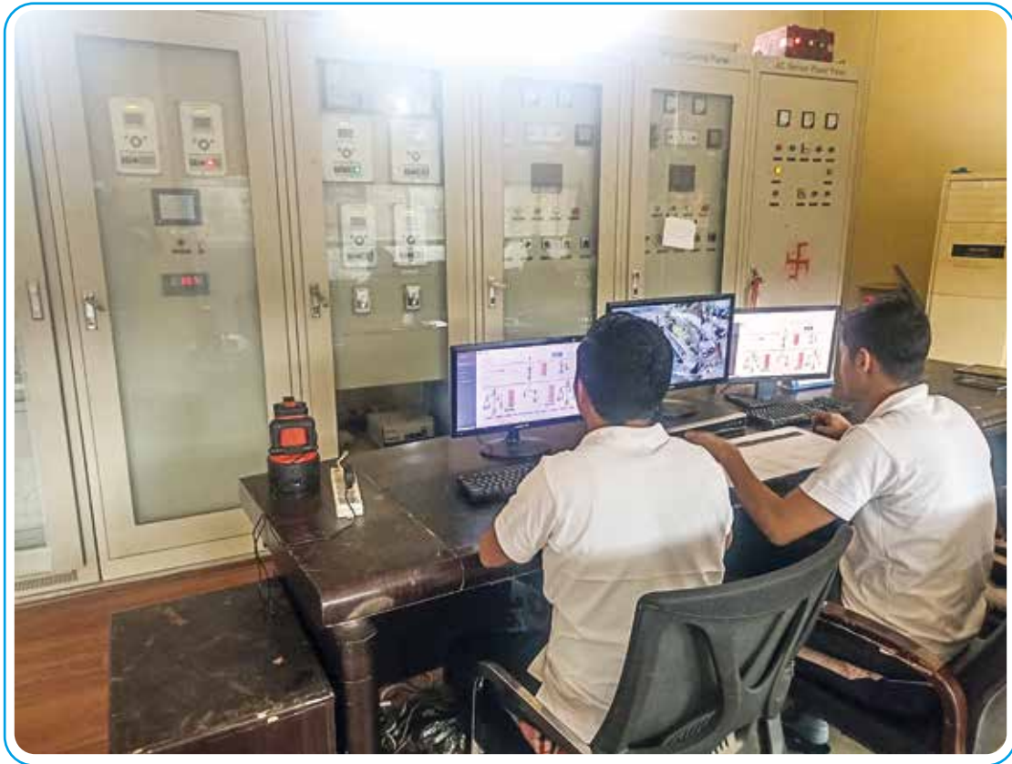
Powerhouse Control Room of Tadi Khola HEP
