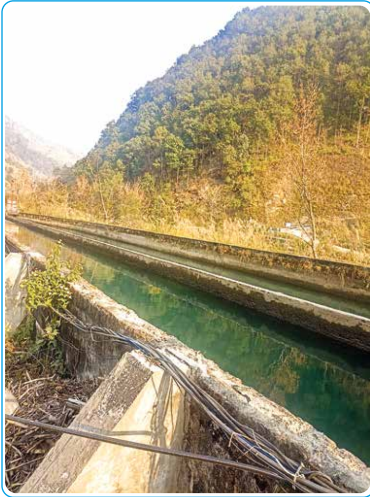
Desanding Basin of Tadi Khola HEP
