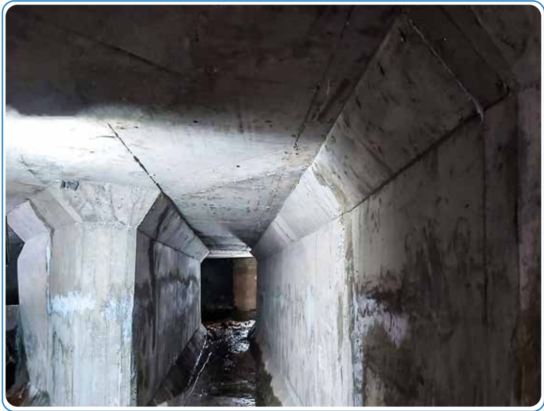
U#1 Tailrace culvert- inner side of Mistri Khola HEP
